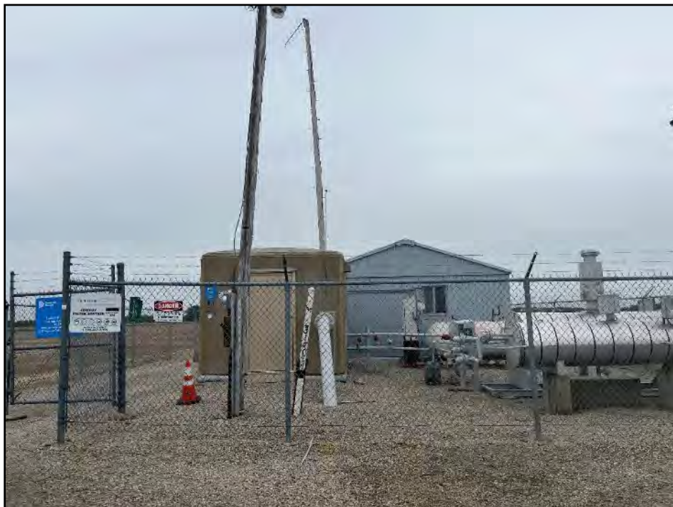
Photograph 4. Convoy M&R Station, located south of Convoy Road in the western portion of the project area, is a public utility development within the project area.
