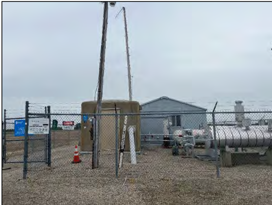
Photograph 4. Convo M&R Station, located south of Convo Road in the western portion of the study area, is a public utility development within the study area.
