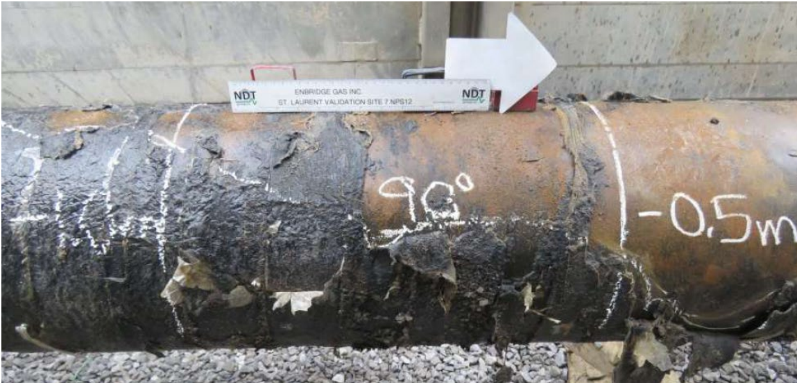
Figure 5: Dig Site 7 - Coating Damage
