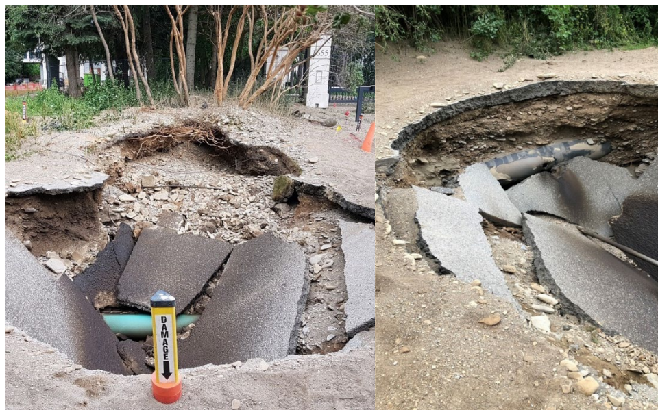
Figure 16: Pipeline Failure on NPS20 Distribution Main Operating at 175psi – Detailed
