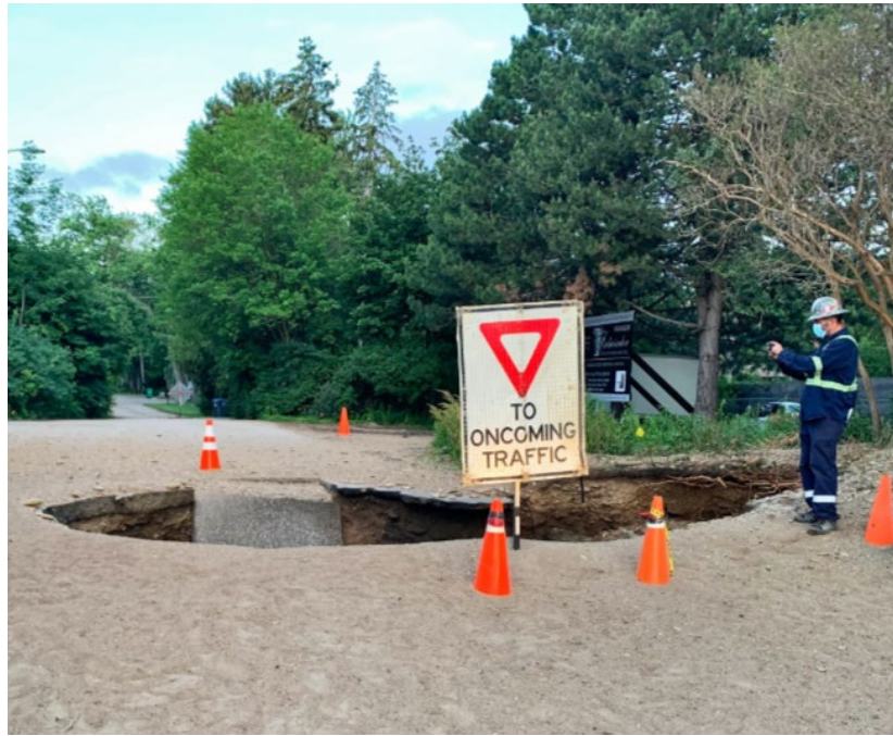
Figure 15: Pipeline Failure on NPS20 Distribution Main Operating at 175psi – Site Overview
