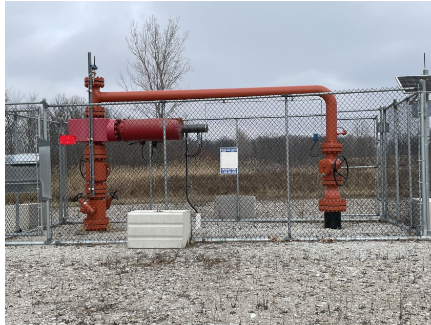
Image 1. Typical Injection – Withdrawal Well Wellhead
