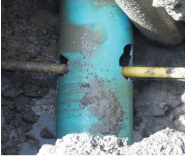
Image: Example of a cross bore
