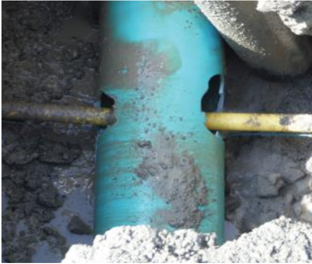
Image: Example of a cross bore
