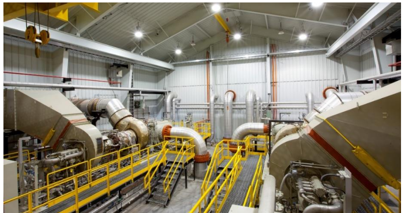
Image: inside a building housing a compressor station
