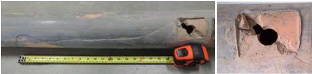
Figure 5.2-41: Rapid crack propagation on Aldyl A pipe from saddle tee fusion (Mississauga, ON)
