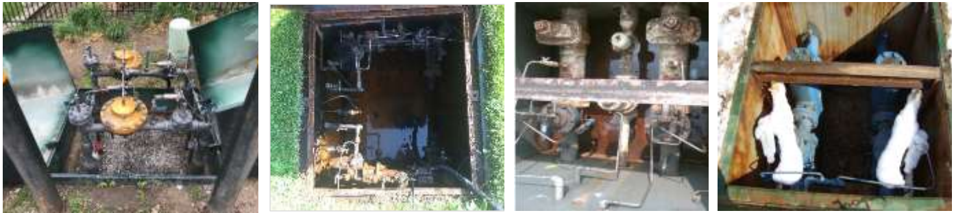
Figure 5.3-6: Examples of Distribution System Stations
