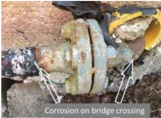
Figure 5.2-7: Severe corrosion on bridge crossing pipe
