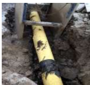
Figure 5.2-25: Gouges and dents due to latent damages
