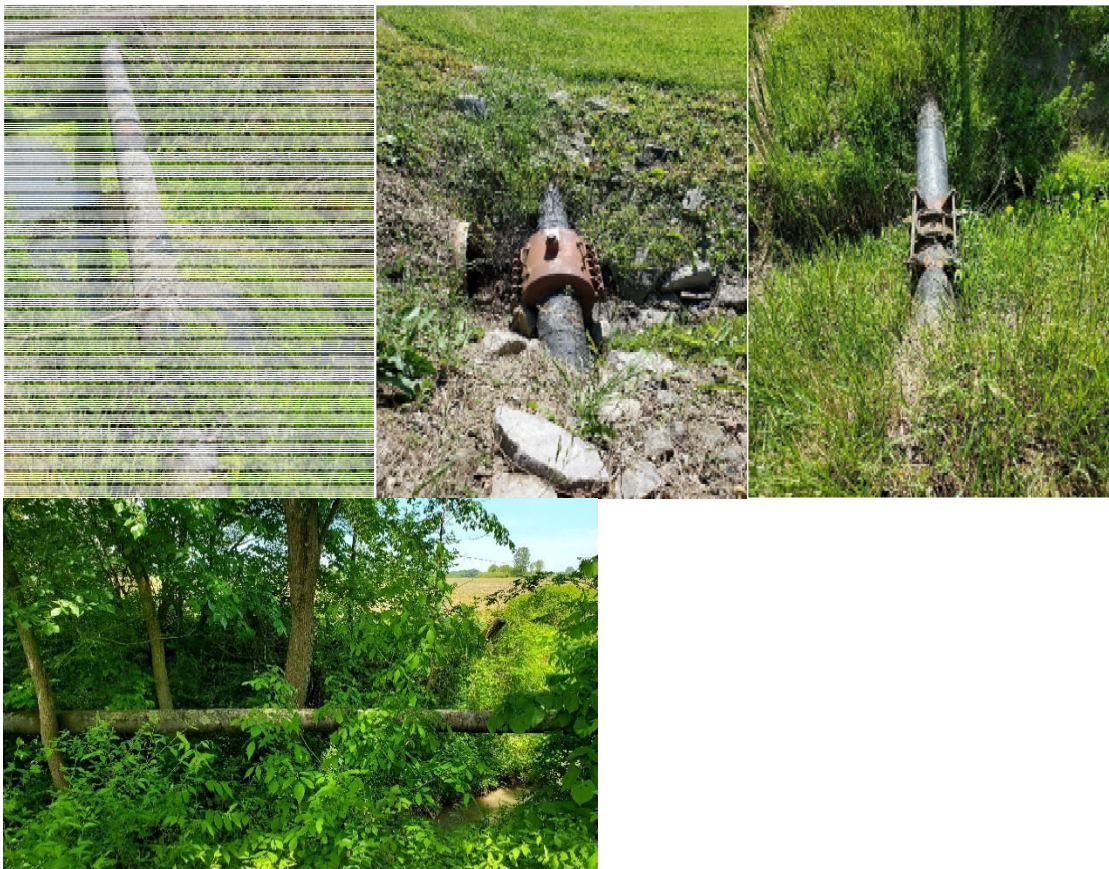
Figure 4-1 Examples of London Lines Exposed Piping (June 2020)
