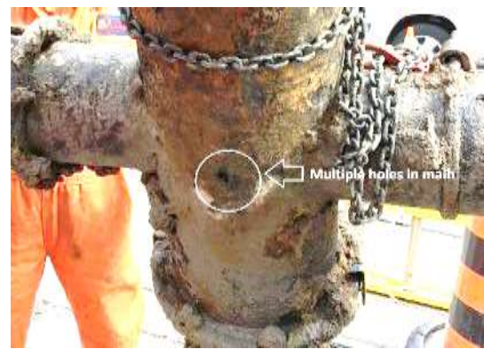
Figure 5.2-18: Multiple leaks on vintage NPS 12 gas main
