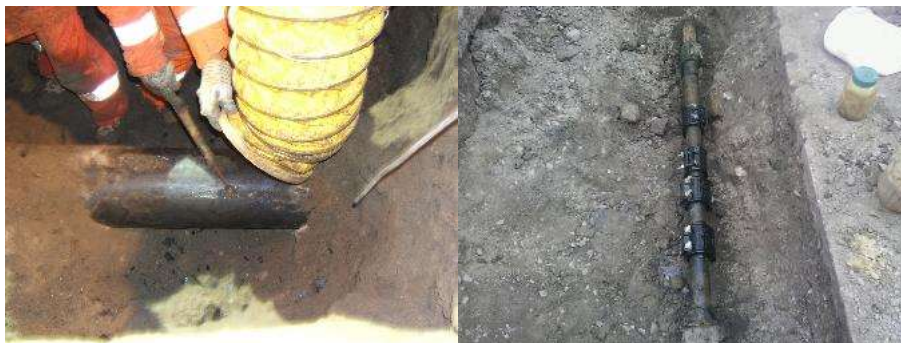
Figure 5.2-34: Bare and unprotected steel failures
