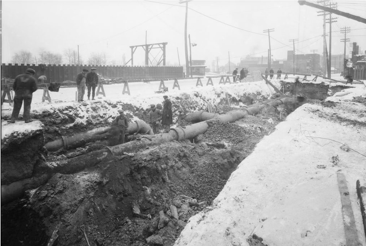
A photo taken in 1926 of the construction of a gas pipeline from Eastern Avenue to Don Roadway in Toronto.
