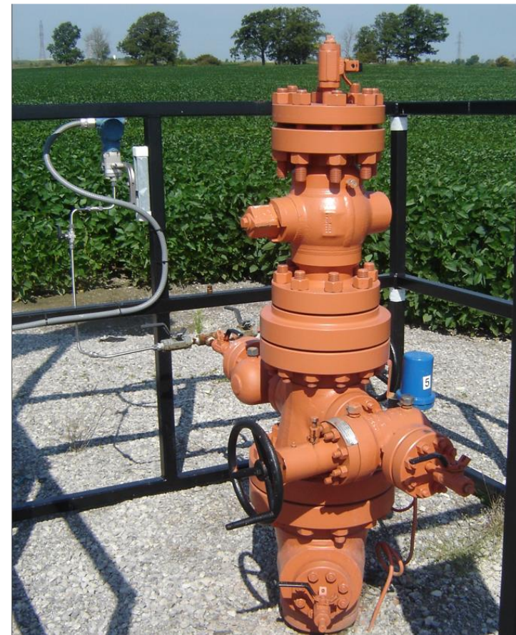
Photo 2. Photo of a typical wellhead configuration for an observation well
