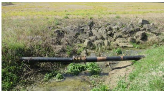
Figure 5.2-13: Aerial crossing with exposed mechanical fitting
