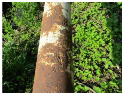
Figure 5.2-14: Coating degradation and corrosion pitting
