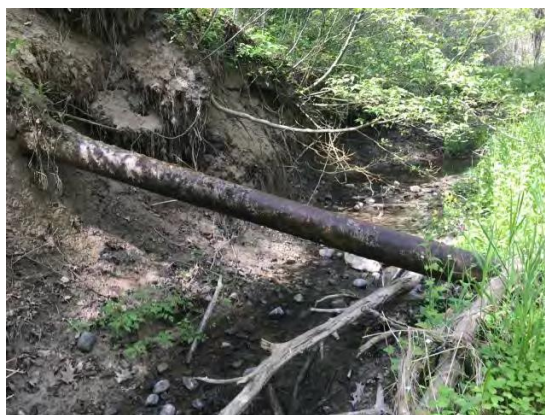
Figure 5.2-15: Erosion increasing the unsupported length of an aerial crossing
