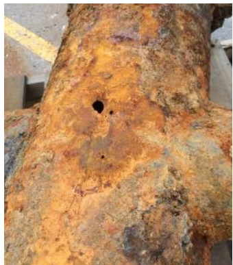
Figure 5.2-24: Multiple leaks due to severe corrosion on vintage NPS 12 gas main
