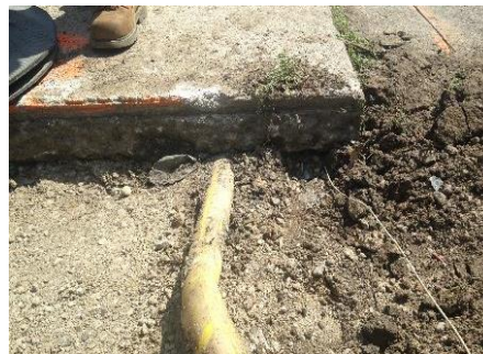
Figure 5.2-8: Shallow and embedded gas main due to road grade change
