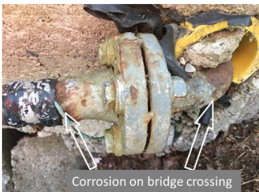
Figure 5.2-9: Severe corrosion on bridge-crossing pipe
