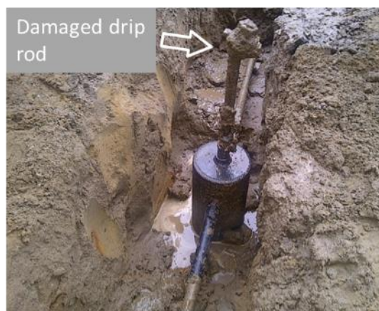
Figure 5.2-12: Damaged drip rod on vintage NPS 2 gas main
