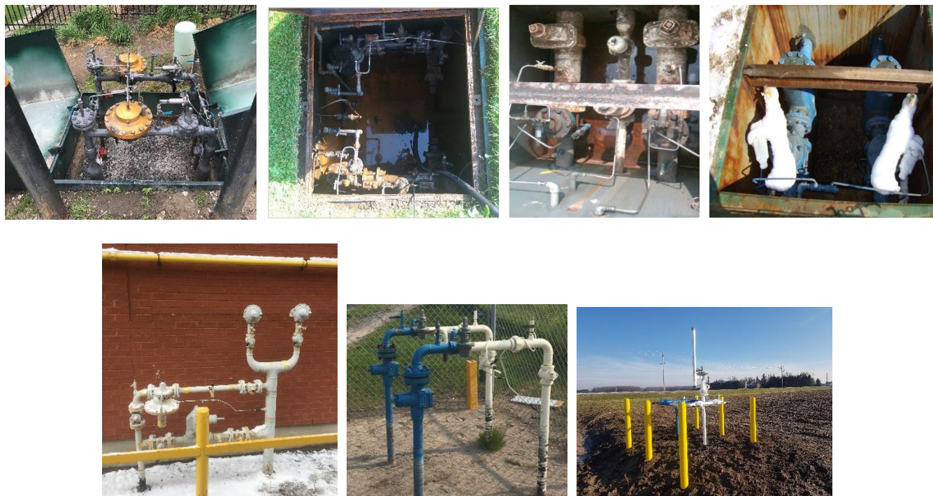
Figure 5.2-66: Examples of Distribution System Stations
