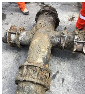
Figure 5.2-23: Detail of fabricated fitting after removal
