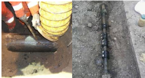
Figure 5.2-7: Bare and unprotected steel failures
