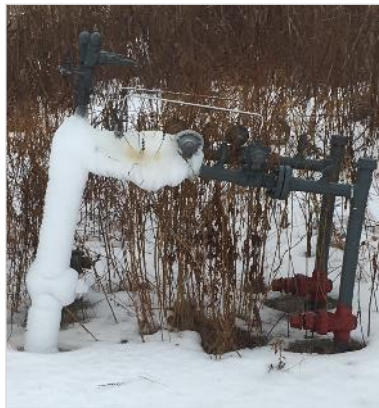
Figure 5.2-68: The Joule-Thomson Effect on a District Station
