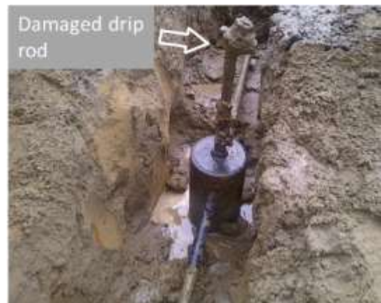
Figure 5.2-10: Damaged drip rod on vintage NPS 2 gas main
