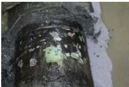
Figure 5.2-24: Multiple corrosion sites on NPS 12 St. Laurent pipe
