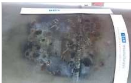
Figure 5.2-20: NPS 20 KOL pipeline displaying 70% wall loss identified by ILI in 2016
