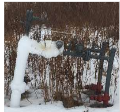
Figure 5.3-9: The Joule-Thomson Effect on a District Station
