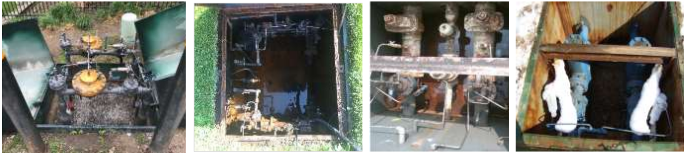
Figure 5.3-6: Examples of Distribution System Stations
