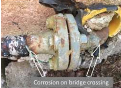
Figure 5.2-7: Severe corrosion on bridge crossing pipe
