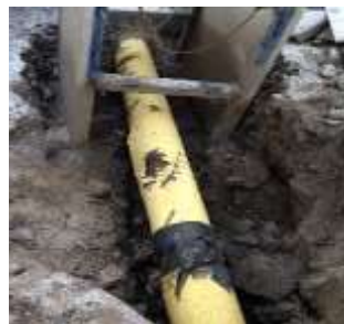
Figure 5.2-25: Gouges and dents due to latent damages
