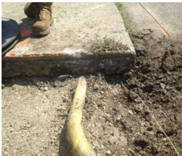
Figure 5.2-6: Shallow and Embedded Gas Main due to Road Grade Change
