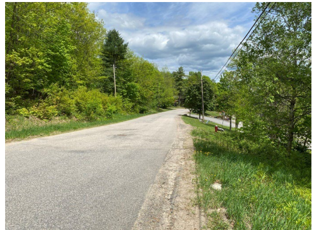
Photo 4: Steep embankment, slope in excess of 20°, looking east along Hidden Valley Road
