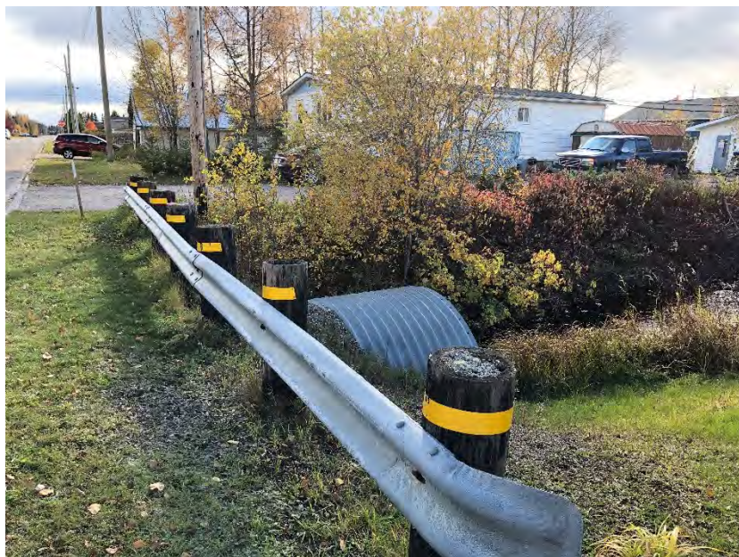
Photo 10: Disturbed area due to ditching and culvert installation – not surveyed, facing southwest
