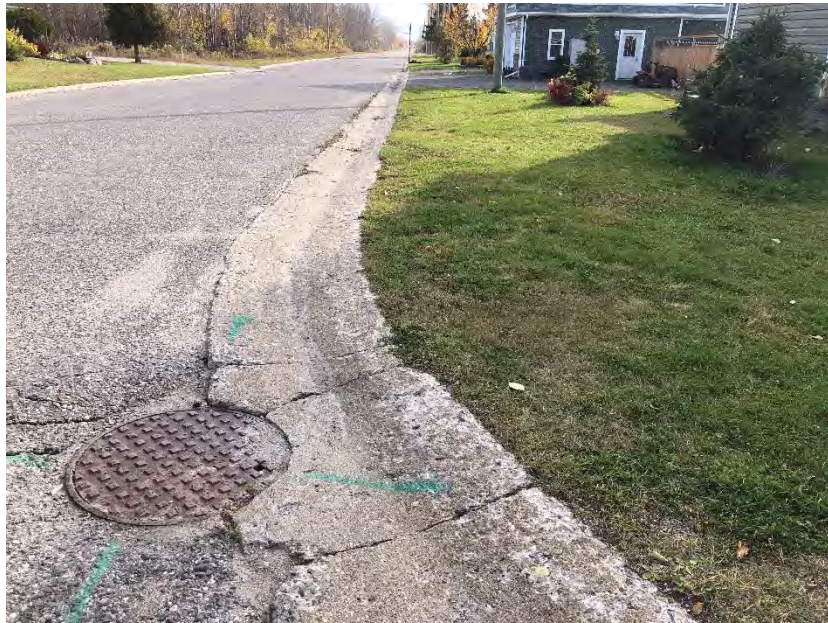
Photo 9: Disturbed area due to the installation of buried utilities – not surveyed, facing southwest
