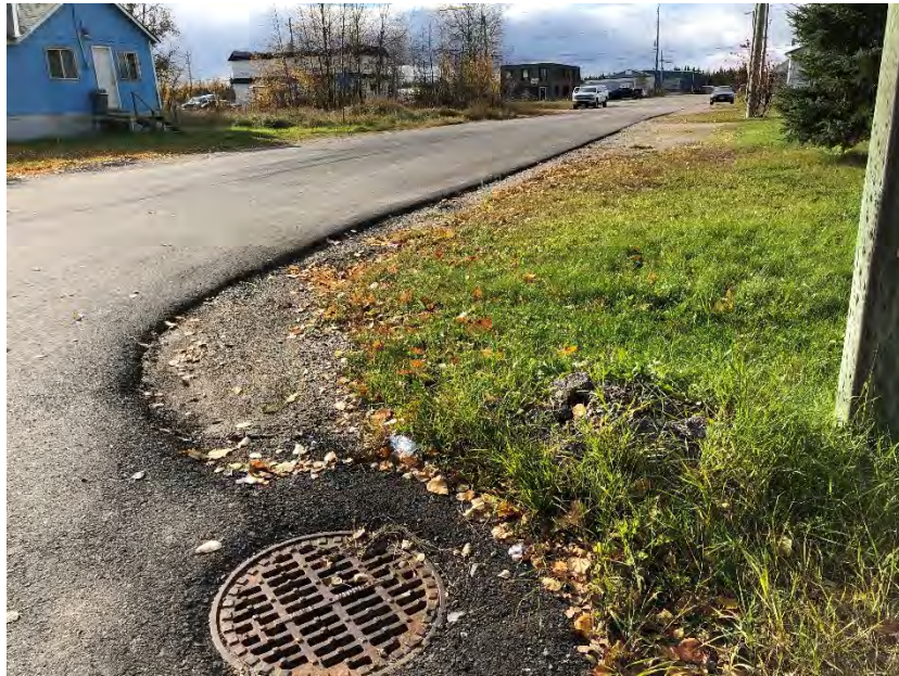
Photo 11: Disturbed area due to grading for road and utility installation – not surveyed, facing west
