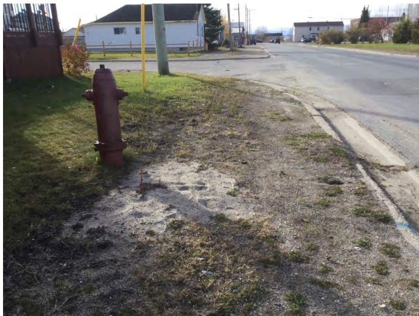
Photo 8: Disturbed area due to the installation of buried utilities – not surveyed, facing south
